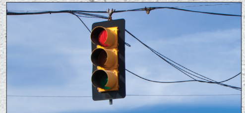
Broken cable ties and lashing wire are a common headache for municipalities.
